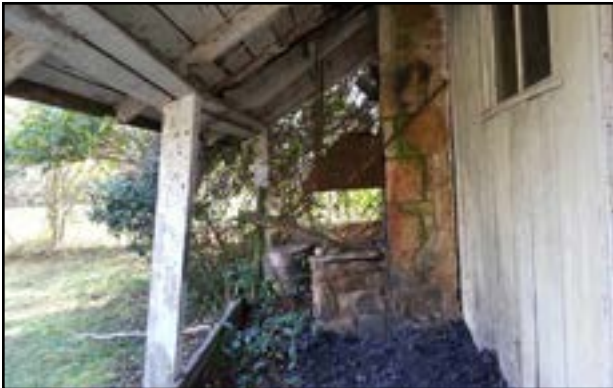
Dilapidated shop in October 2014. Photo by Karen Stone.
