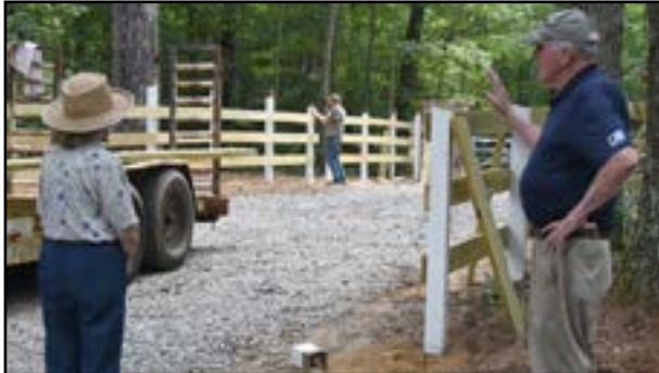
Board members, Karen Stone and Charles Adams, watch as new fencing is installed inside the Taft Highway entrance.
