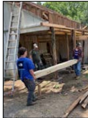
Supervised by volunteer Terry Knox, center, Brooks Barber and Aidan Shakespeare prepare to set a new sill beam.
