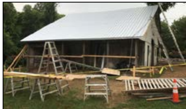
On the south side in July, the new tin roof is apparent. Over 12,000 pounds of cedar shake and asphalt shingles were removed from this side – in addition to 6,800 pounds from the north side. It's no wonder the old roof was sagging.
