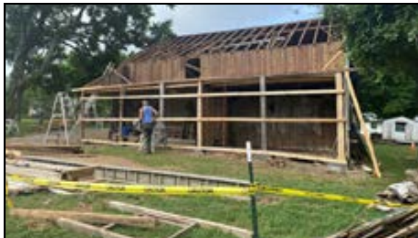
Slim works on the north side of the barn with roof decking and siding removed in June. Two interior spaces are visible.
