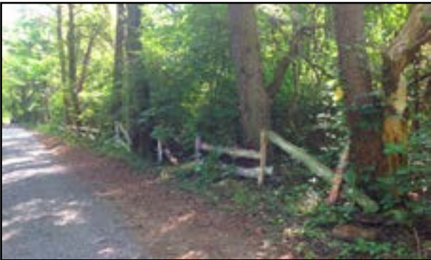
Deteriorated state of the back drive fence on July 1, 2019.
