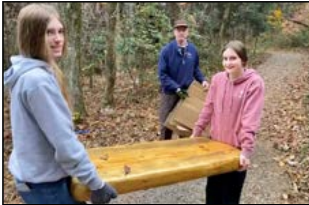
Maggie and Lily help Andy Jones install a bench on the trail.
