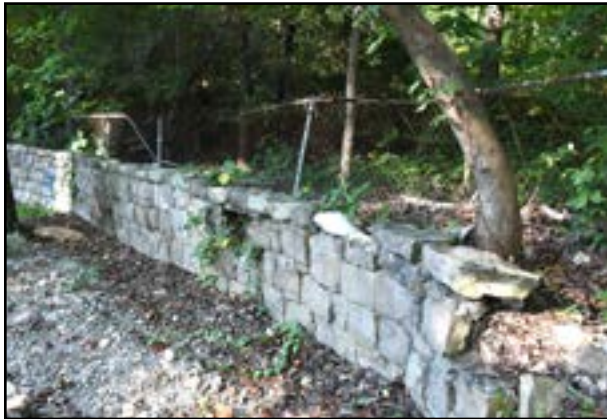
The damaged cut-stone wall at the Emma Bell Miles homesite will be repaired with a grant from the Tucker Foundation.
