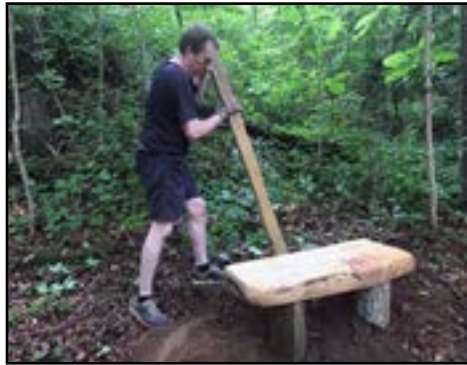
Andy Jones tamping earth to seat a new bench on the trail. Andy continues the trail bench project with help from Matt
