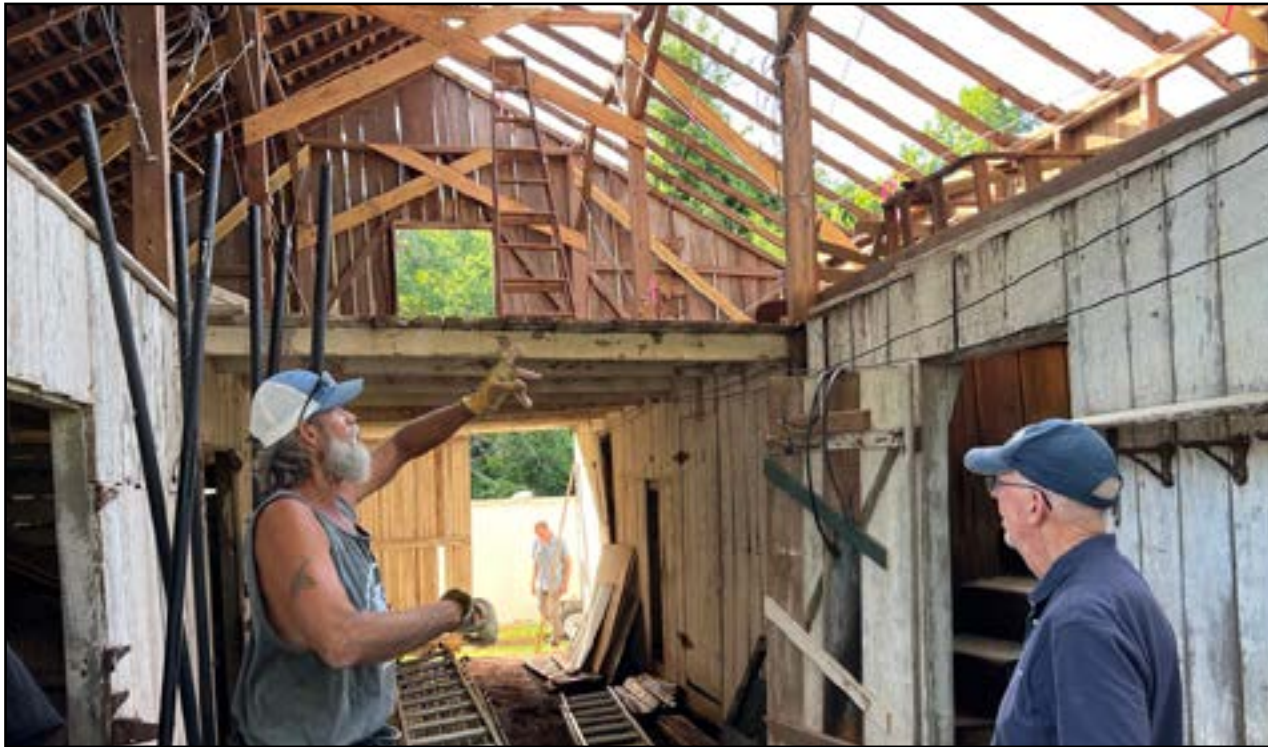
The barn expert, affectionately known as Slim, points out the open rafters to Earl Hereford where 6,800 pounds of asphalt shingles were removed from the north side alone. With the shingles gone, the decking was evaluated and found so deteriorated that it must be replaced. As far as possible, original materials are salvaged and reused so the appearance of the barn is preserved.
