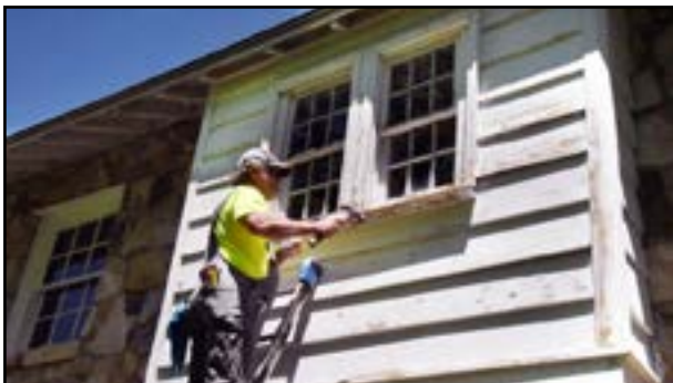
At the Carriage House, craftsman David Clark is pulling out the old window sashes, repairing, and replacing them. He has also repaired and painted siding, soffits, and woodwork on the exterior and on the balcony. Photo by Charlie Stone.
