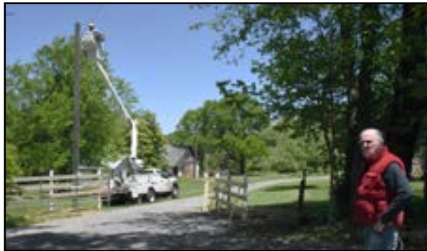
Board Projects Chairman, Charles Adams, watches from a safe distance as a lineman for EPB installs and directs new LED lighting fixtures for the parking lots. The new lights will be closer to the ground and directed downward to provide needed security while making as little impact as possible on the night skies and the neighbors. Photo by Charlie Stone.
