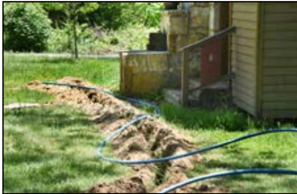
New water lines are going into the Pavilion. This will not only improve water pressure but also allow for easier winterizing of the lines. Photo by Charlie Stone.
