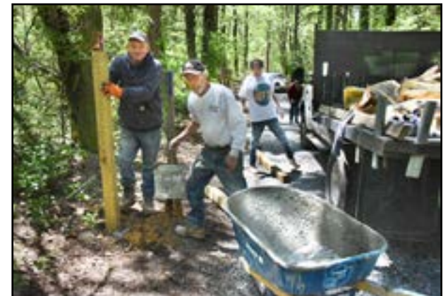
Mark Turner, owner of Middle Valley Fence Company, holds a post in place while Paul Patterson fills the base with concrete. Malcolm Turner assists in related tasks. Photo by Charlie Stone.
