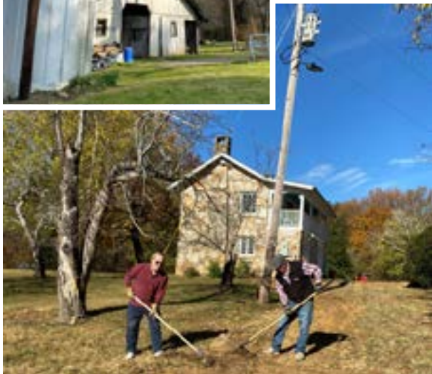
Below, volunteer David Reed and Earl Hereford fill in the ditch over newly buried lines.
