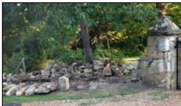
Stonemason Randall Hawkins numbered each stone as he removed it so he could rebuild the wall as much like the original as possible. Photo taken by Gene Adams, August 5, 2019.
