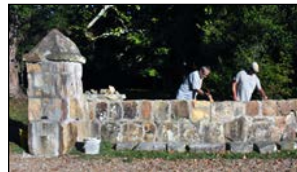
Randall and his son, Parker, are shown preparing to add the capstones. Randall's brothers, Abe and Claude David, had repaired the wall before. Photo by Charlie Stone, August 15.
