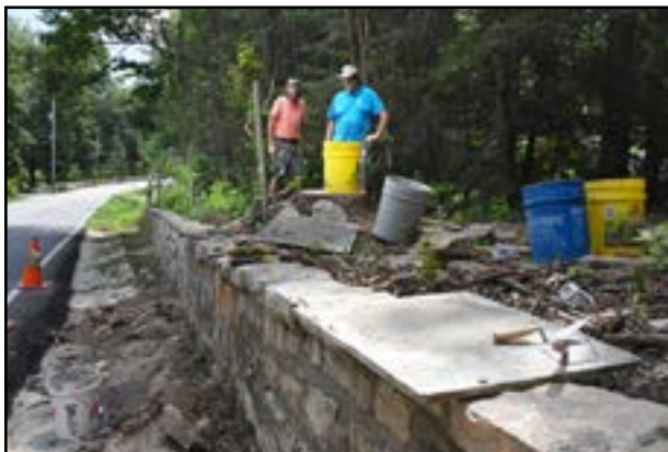
Many have stopped to admire the craftsmanship and to thank Jayke Hawkins, left, and his father, Randall, right, for their skill in shaping the stone as they restore the wall.
