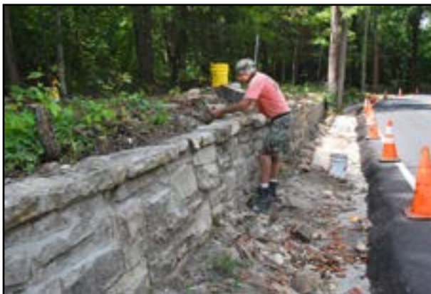
Jayke Hawkins replaces stones in the wall that bounds the Emma Bell Miles homeplace at the corner of Anderson and Taft. A grant from the Tucker foundation financed the work.
