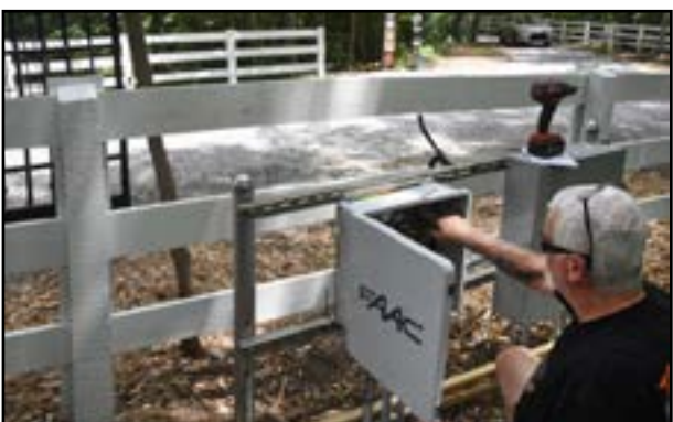
Chuck Lambert sets up the controls for the new Taft Highway security gate. The gate is operated electronically, so it can be opened and closed for the regular visiting hours of dawn till dusk, and no one will be locked in accidentally.
